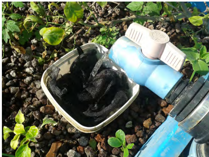
Fig. 4.50 Solids Removal Device in Media Bed Unit
