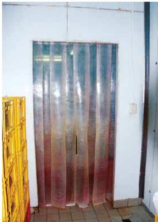
Photo A.4.1 Plastic strip curtain installed in a doorway to reduce entry of warm air
