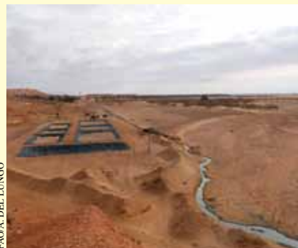
The phytodepuration facility at the Brézina Oasis, which is being installed with the support of the University of Tuscia
