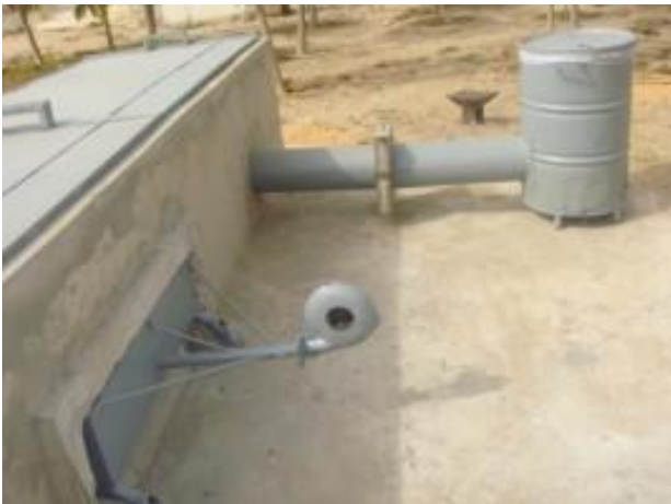
BACK VIEW connected by metal pipe to the external generator via the filter
