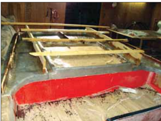
Figure 119 Final stage of the making of the mould for the aft deck.
