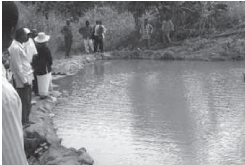
Fig. 5.2. Dam constructed by community members in Mangochi district, Malawi, with technical assistance sourced locally through the project.
