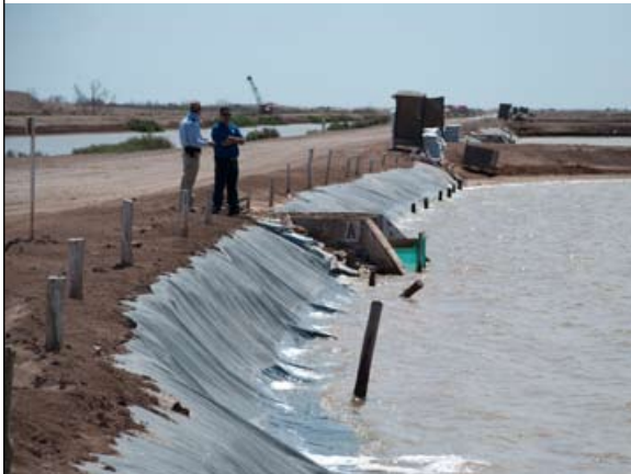
PHOTO 27 Bottom PVC lining in an earthen pond
