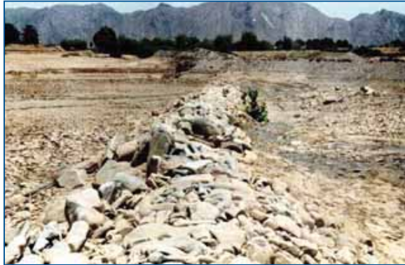
FIGURE 4.7 Partially breached diversion spur in Wadi Beihan (viewed from the wadi towards the canal intake)
