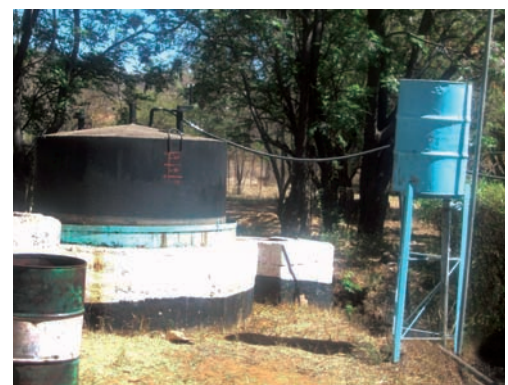
Gas collection tank resting on the concrete-built digester. Pipes / tubes at the top of the gas tank supply the house with methane gas, Botswana. (Reuben Sebegu)
