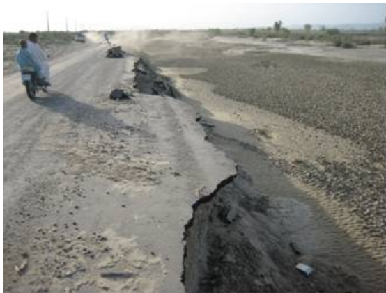
Figure 3.32 Damage caused by Cyclone Gonu in the Islamic Republic of Iran Source: Zahmatkeshan and Saadatkhah, 2007.
