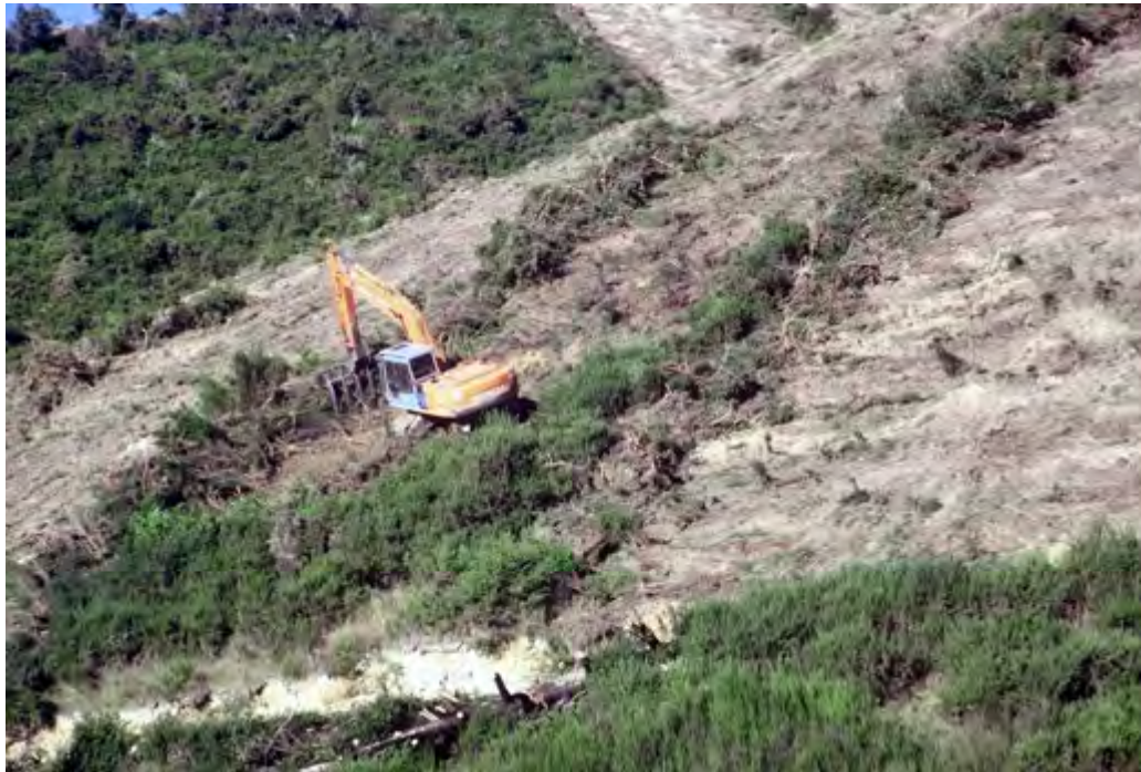
FIGURE 8.5 Windrows made using a backhoe with a root-rake attachment. Note that there is some soil disturbance.
