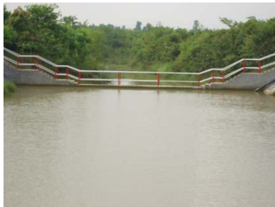
Fig.10. Water control structures across the canals to conserve water
