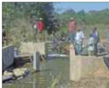
Lubumbashi. A catchment basin (top) at Kaluako, north of the city, provides irrigation water throughout the year. Above, a water control structure nears completion on a stream at Kilobelobe
