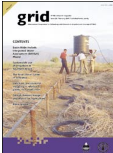
Installation of low pressure drip irrigation close to Makanya, Tanzania. (FAO/V. GILLET)
