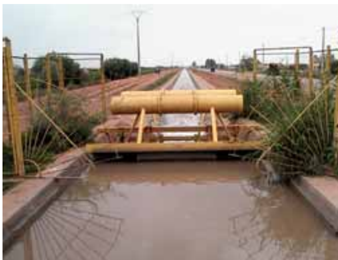
Plate 6 A self-acting upstream control gate (AMIL gate).
