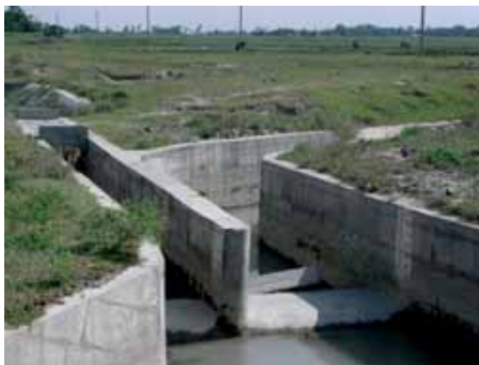
Plate 1 Proportional fixed divider structure seen from upstream, SMIS, Nepal.
