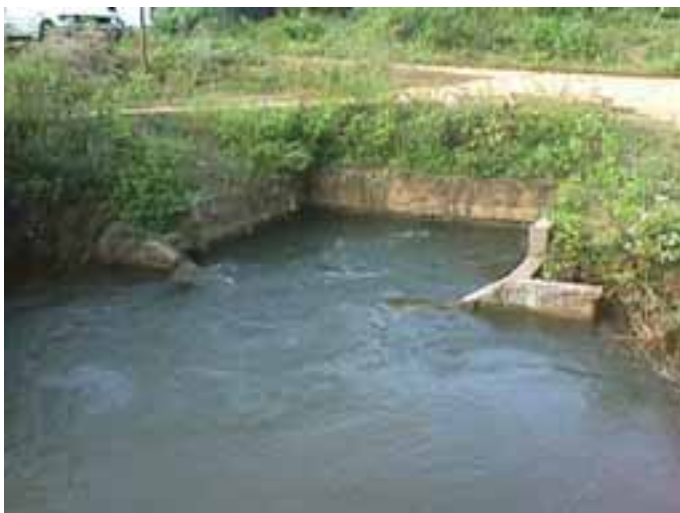
Plate 16 Offtake with downstream submerged conditions.
