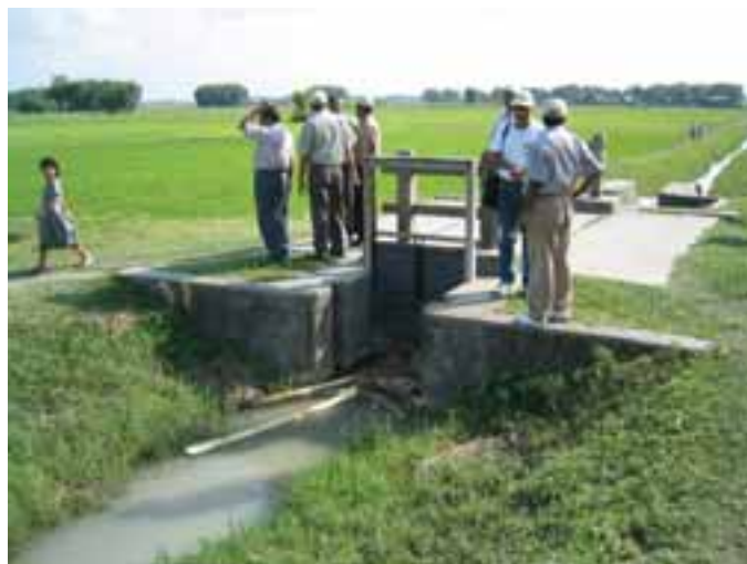
Plate 12 Dysfunctional cross-regulator (spindle missing) along a secondary canal, SMIS, Nepal.
