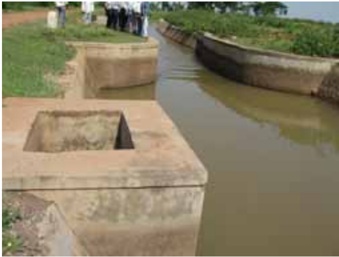
Plate 20 Measurement capacity: submerged flume with no critical section, yielding incorrect measurements GLBC, Karnataka, India.
