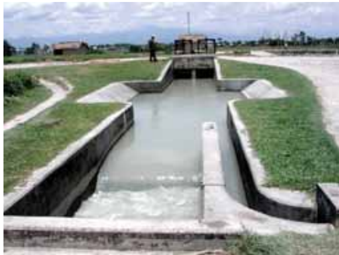
Plate 18 Dysfunctional proportional divider (Nepal) with different downstream conditions: free-flow (main branch left) and submerged (small branch right). The capacity of the structure with respect to proportional division is at stake.
