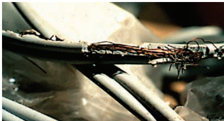
damage to cable
