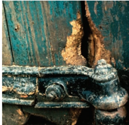
damage to structures
