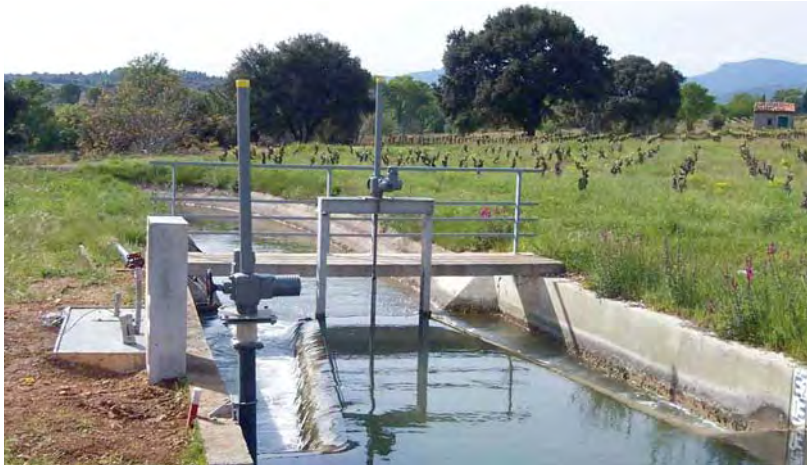
Figure 1. Control structure with motorized gates.
