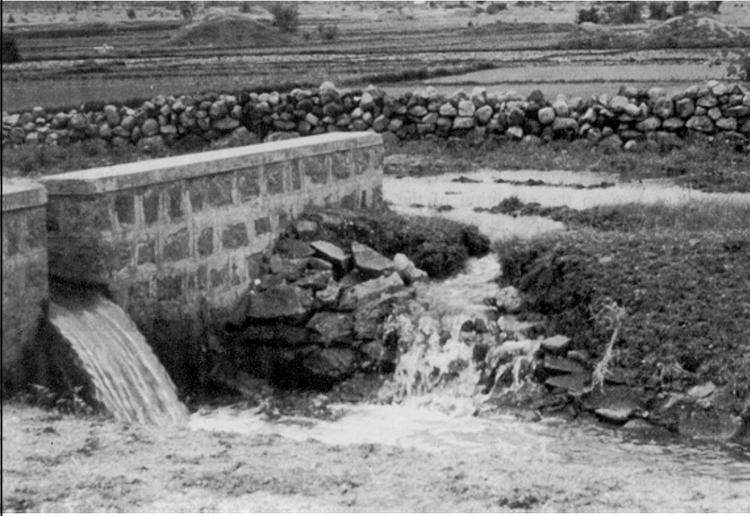
FIGURE 51 Leakage around a structure
