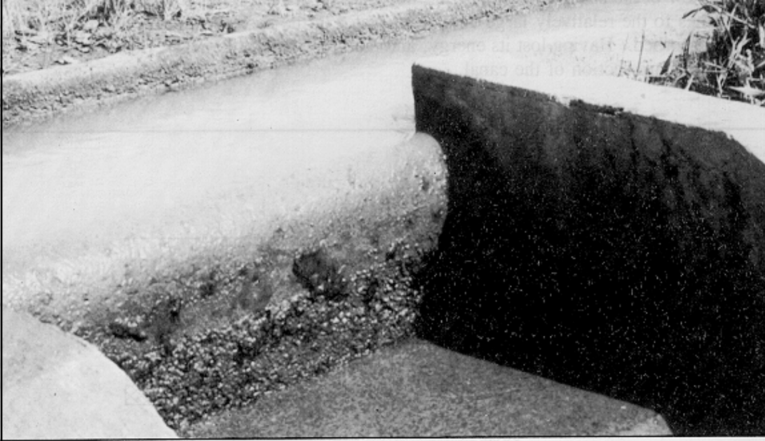
FIGURE 42 Spillway or emergency outlet
