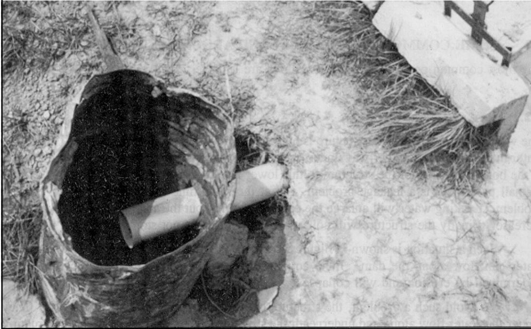
FIGURE 54 Leakage that resulted in erosion
