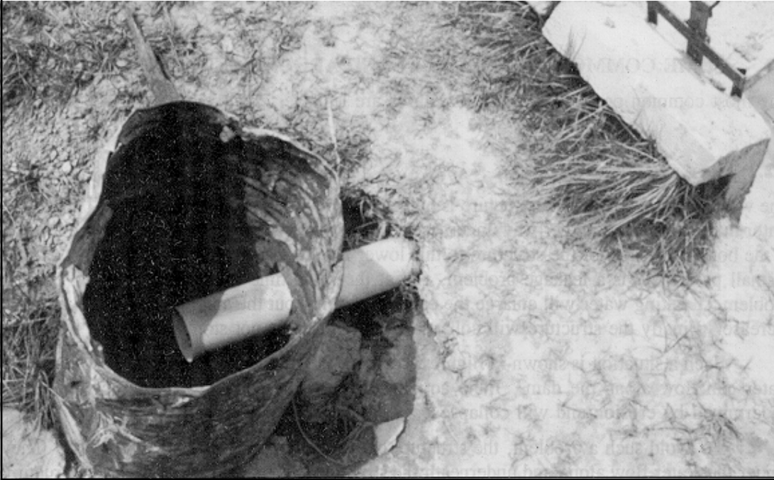
FIGURE 54 Leakage that resulted in erosion
