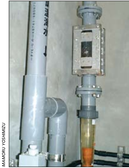
Figure 6.5: Electrolyzer with flow meter used for oyster depuration
