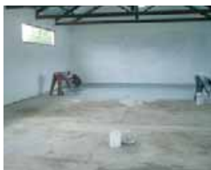
A new concrete floor was laid and sealed with epoxy resin for chemical resistance.
