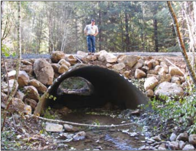
A rebuilt culvert in the Umpqua National Forest, Oregon: many Forest Service projects funded under the American Recovery and Reinvestment Act are designed to improve water quality and restore critical fish habitat and passage
