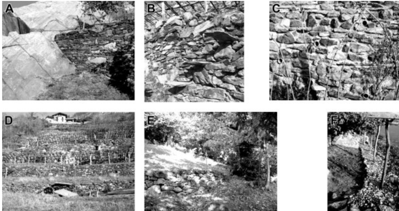
Fig. 2 Terraced slopes in Valle d'Aosta. Structural typologies and details (Photos M. Freppaz). a) wall foundation; b) connection between terraces (suspended stairs); c) example of restored wall; d) terraced slope – vineyard; e) terraced slope – chestnut wood
