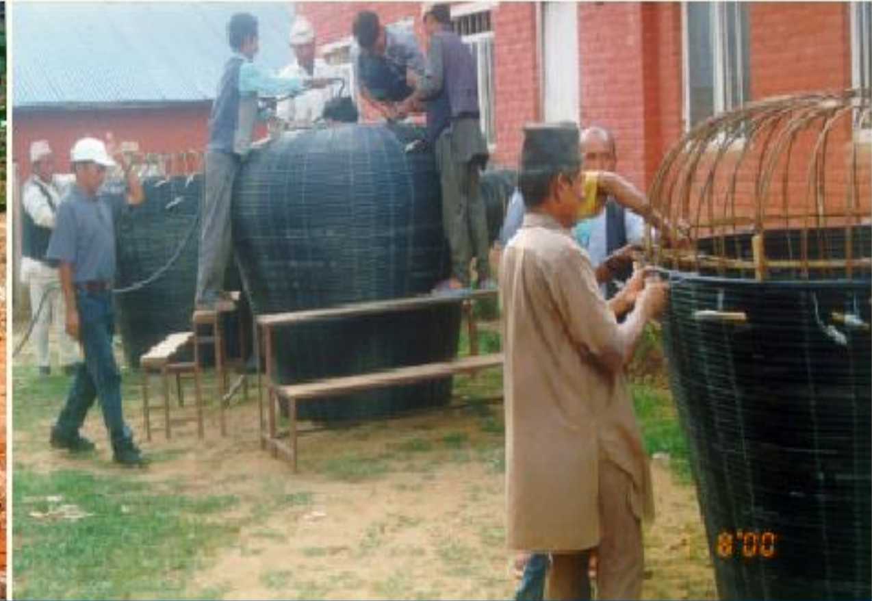
Roofwater storage system for drinking water use and for low cost drip irrigation during dry season. For cash crop production (Nepal)
