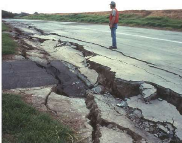
Figure 12. Photograph of lateral spread damage to a roadway as a result of the 1989 Loma Prieta, California, USA, earthquake. (Photograph by Steve Ellen, U.S. Geological Survey.)
