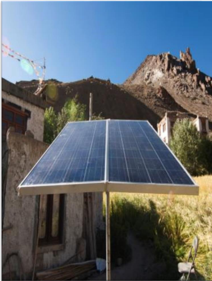
250 -500 W Solar DC Grid
