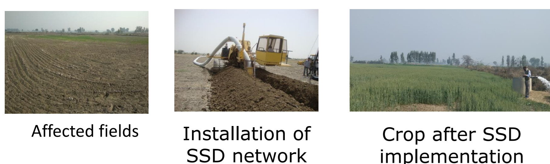
Fig 2. View of affected site in winter, installation of SSD network and pumping of drainage effluent
