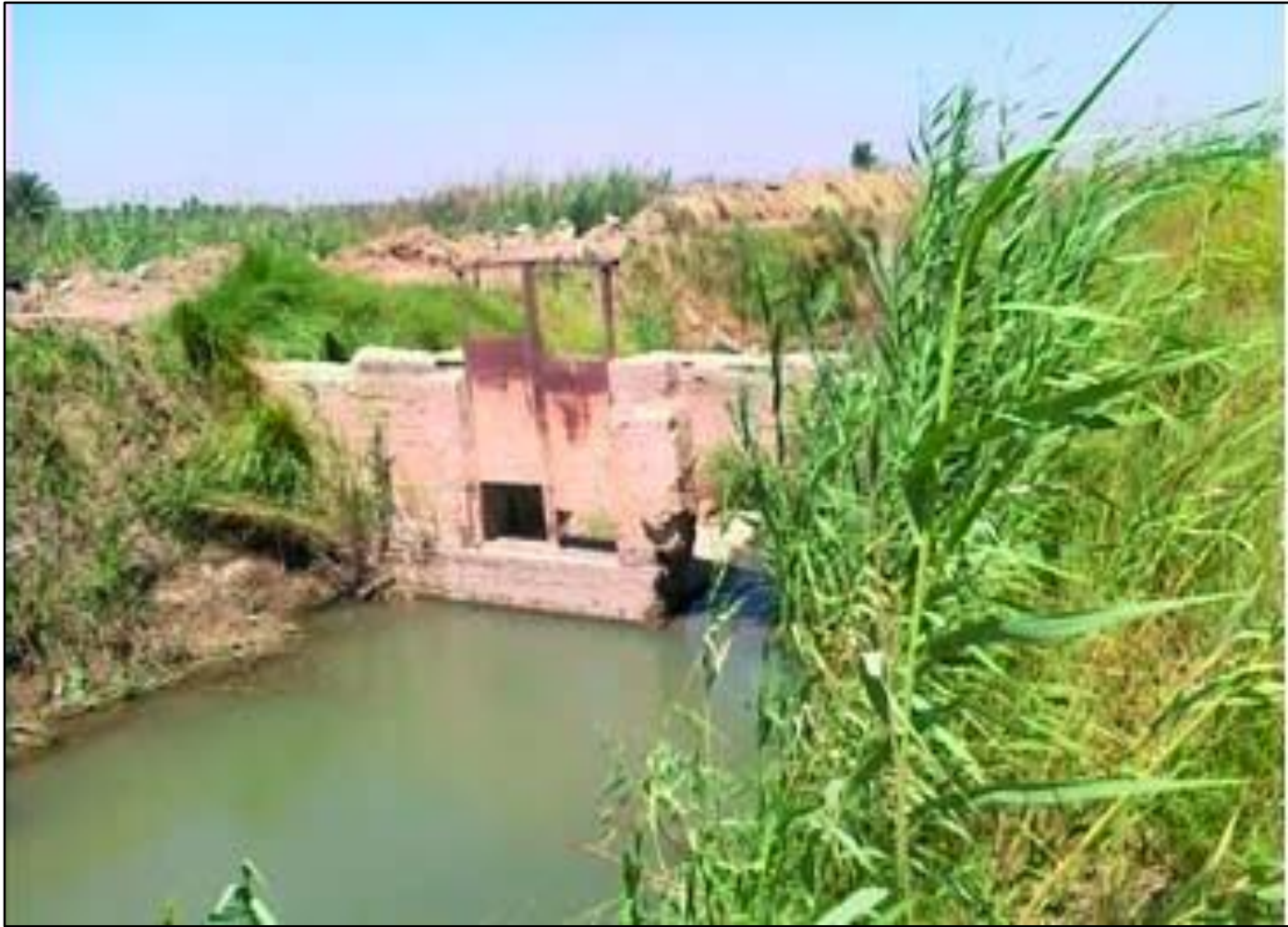
Loss of the formal shape of a major irrigation channel in the Musayyib irrigation project
