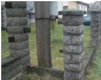
Improper use of land
