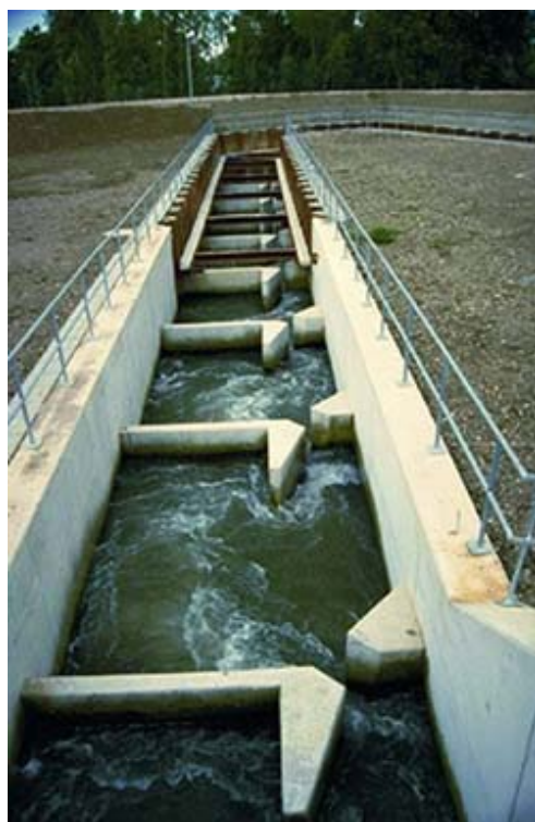
Photo 5: The vertical slot fish pass at the Iffezheim dam is an example of a recently built fish pass facility on the river Rhine. Together with the sophisticated entrance construction (i.e. several entrances to attract fish towards the pass), the 37 pools help fish to pass the 10 m high obstacle (Photo: M. Larinier).
