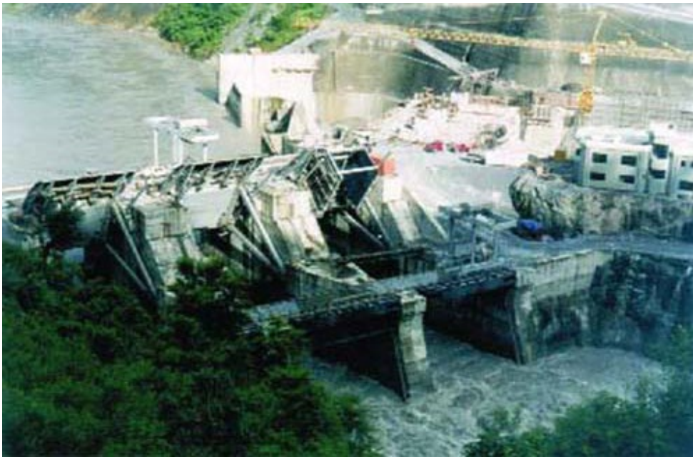
Photo 2: The dam of the Kali Gandaki "A" Hydroelectric Project in Nepal (still under construction when the photo was taken in July 2001) is a typical example of an obstacle that blocks the migratory route of fish species that are important for the river fisheries as no fish pass was constructed for upstream migration. (Photo: G. Marmulla)
