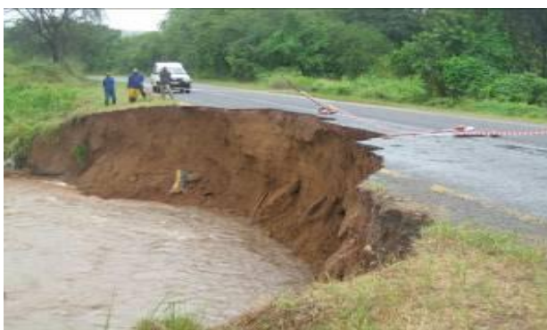
Road under stress from Floods.
