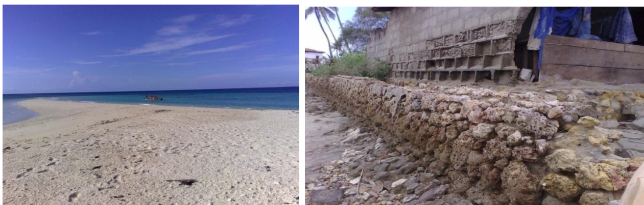
Figure 4. Submerged Maziwe Island, Pangani, Tanga (left) and Collapsing sea defense wall at Pangani Township (right)
